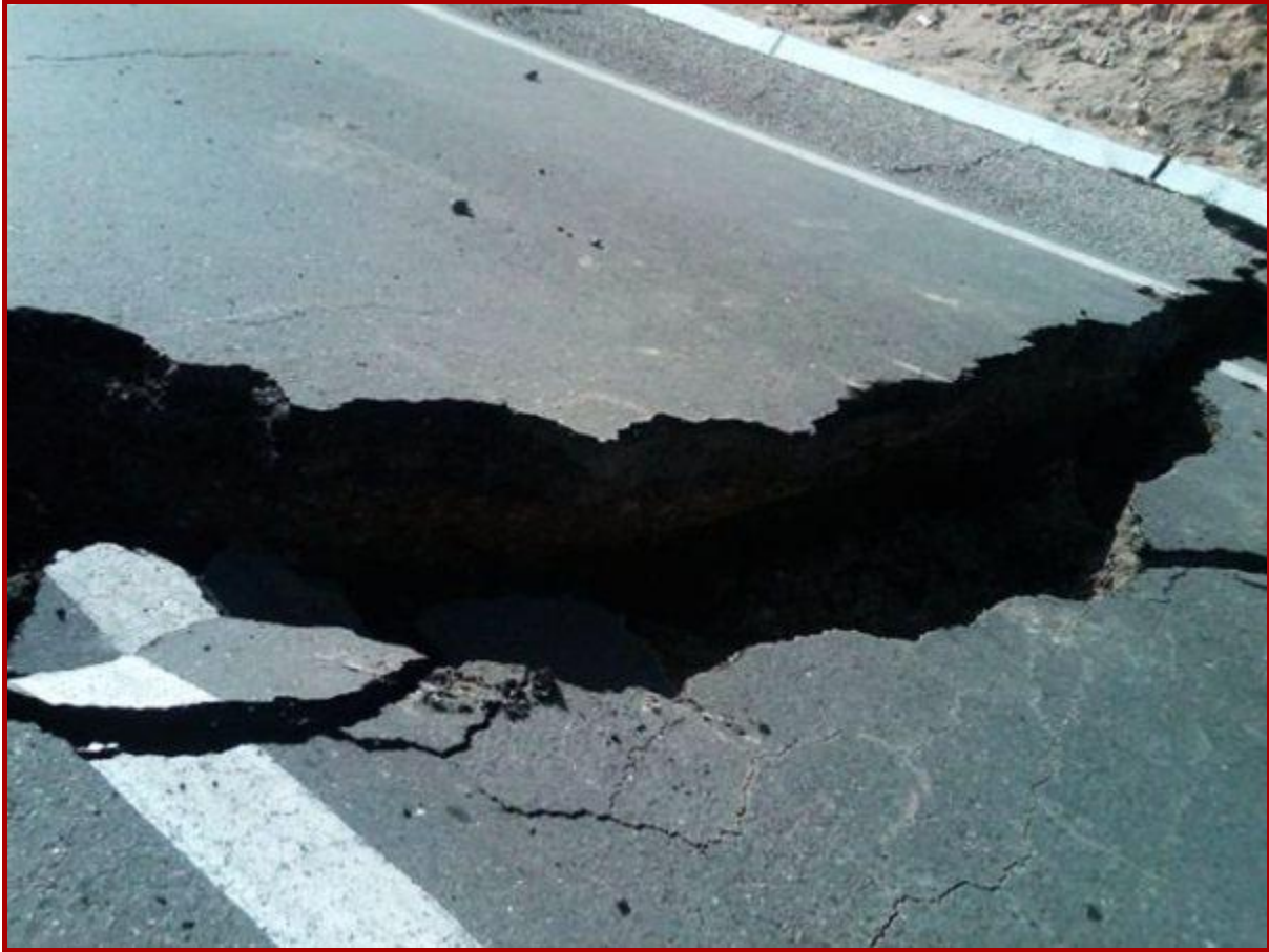
Fig. 24 Structural damage to the Mexicali-Tijuana road at Km 20, near Cerro El Centinela, as a result of the April 4, 2010 earthquake. 24
