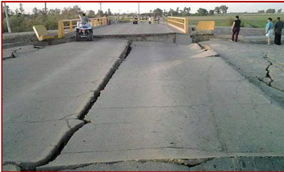
Fig. 23 Structural damage to road and bridge approach in Mexicali, as a result of the April 4, 2010 earthquake. 25
