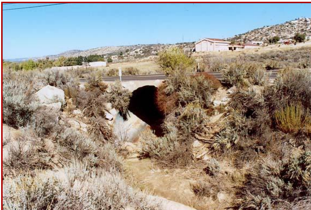
Fig. 17 Culvert crossing at intersection of Campo Creek with State Route 94, San Diego County ( Ponce, 2005 ).
