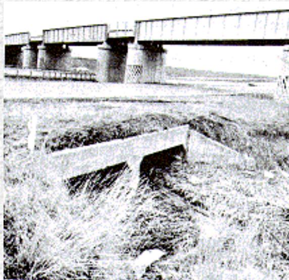
Figure VI-15--Sediment Deposition in Culvert
